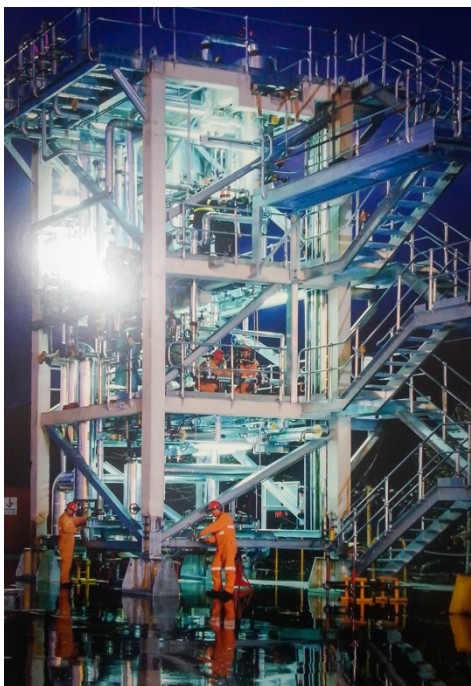
CSR Sugar Treatment Plant – protective coating applied by Cox Steel. Photograph used with permission.
