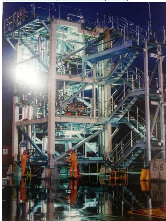
CSR Sugar Treatment Plant – protective coating applied by Cox Steel. Photograph used with permission.
